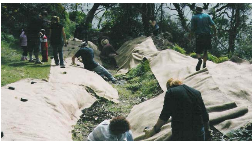
Members of the Bushcare group apply a jute matting to suppress growth of green cestrum seedlings and other weeds. The matting acts as a mulch, retaining moisture in the soil and providing protection for newly planted native plants. Photo: Sutherland Shire Council
